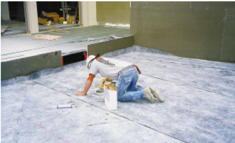
Noble Deck, a sheet membrane engineered for heavy duty exterior applications, was selected for its compatibility with the installation of slate pavers.
