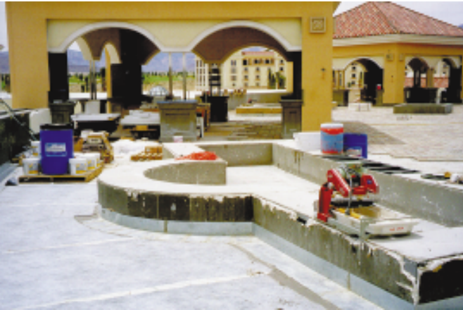
During several points of installation, flood tests were conducted before additional work could commence.
