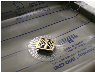
Installed in a full mortar bed method shower with Chloraloy® shower pan liner.
